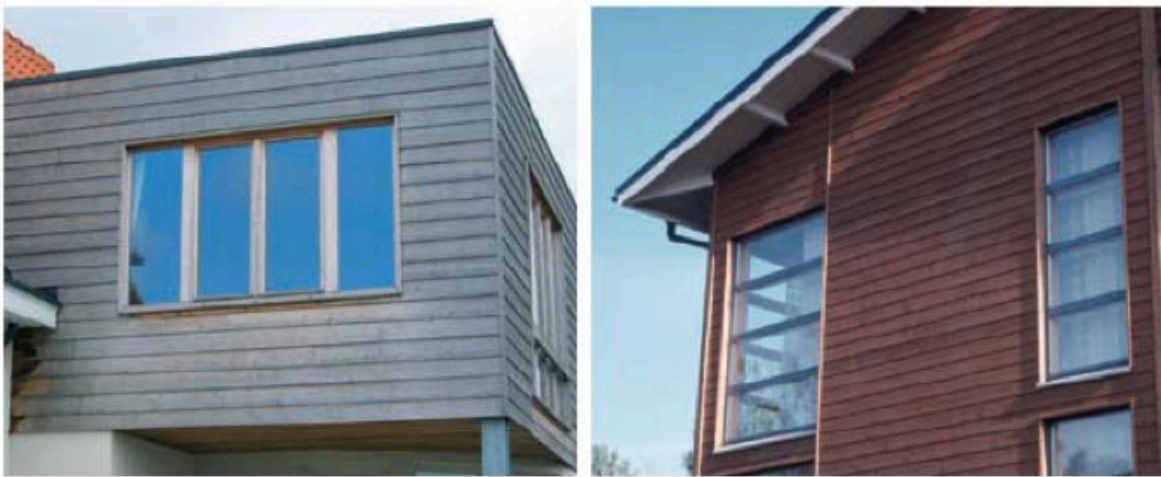
Two examples of ThermoWood cladding after three years weather exposure with and without surface coatings.
